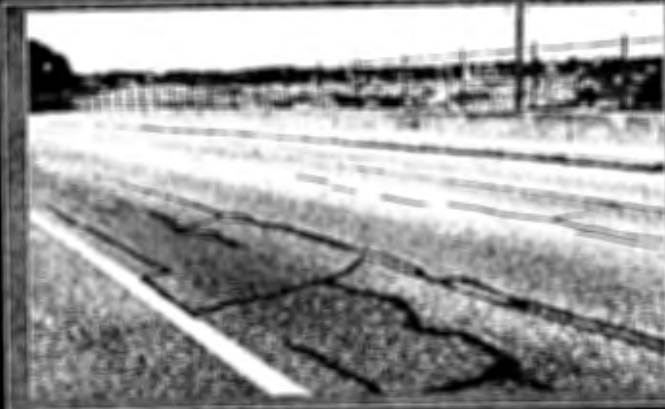
Condition of deck overlay showing transverse and longitudinal cracks.
