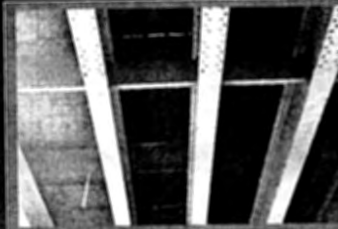
Condition of concrete deck showing random transverse cracks, efflorescence and isolated spalling (Spall is shown).
