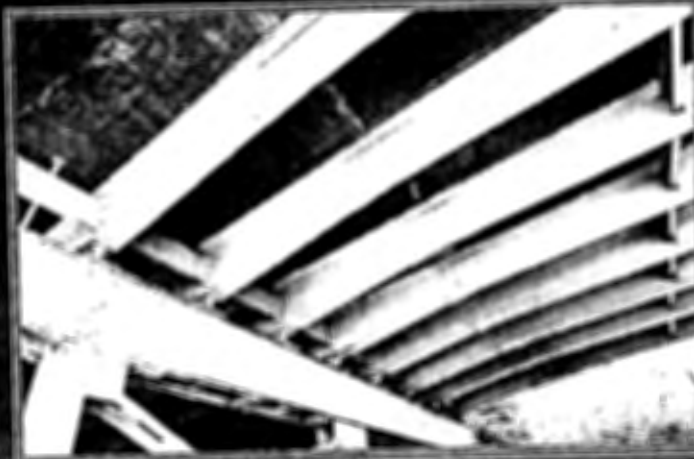
View under Span 8 showing flange transition and field splices adjacent to Pier 6 and 7.
