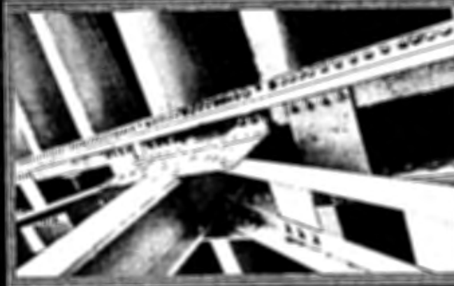
Flange and bottom flange deterioration over center column
